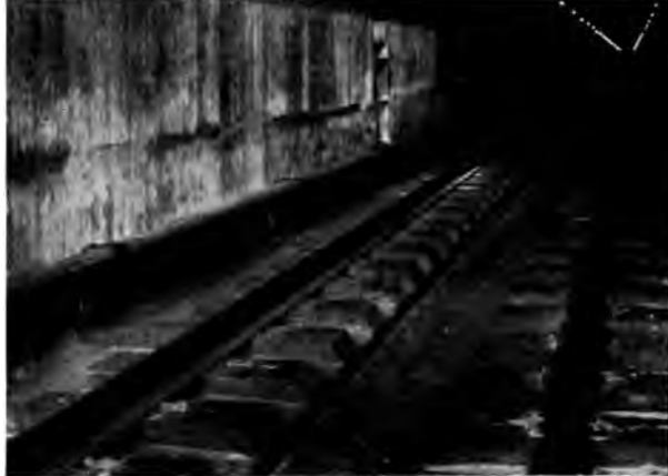
P. & M. Rail Anti-Creepers on the Michigan Central Railroad in the Detroit River Tunnel
